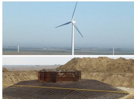
SunEdison's TerraForm Power is acquiring 930 MW of wind capacity from Invenegy, including the Prairie Breeze (top) and under-construction Prairie Breeze II farms (bottom), both in Nebraska. (Source: Invenegy)
